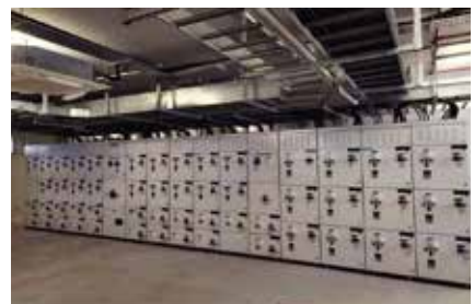
Chemical Plant @ Jurong Island
